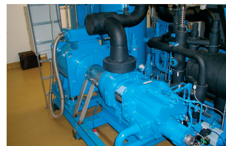
Ethyleneglycol chiller unit
